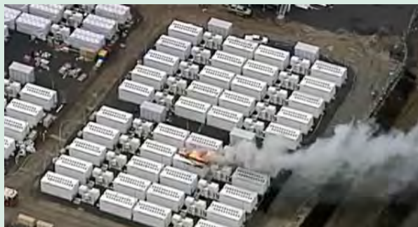
Figure 2: Fire at Victorian Big Battery site near Geelong (Australia) on July 29, 2021. The fire broke out during testing of a battery megapack. Credit: Fire Rescue Victoria
